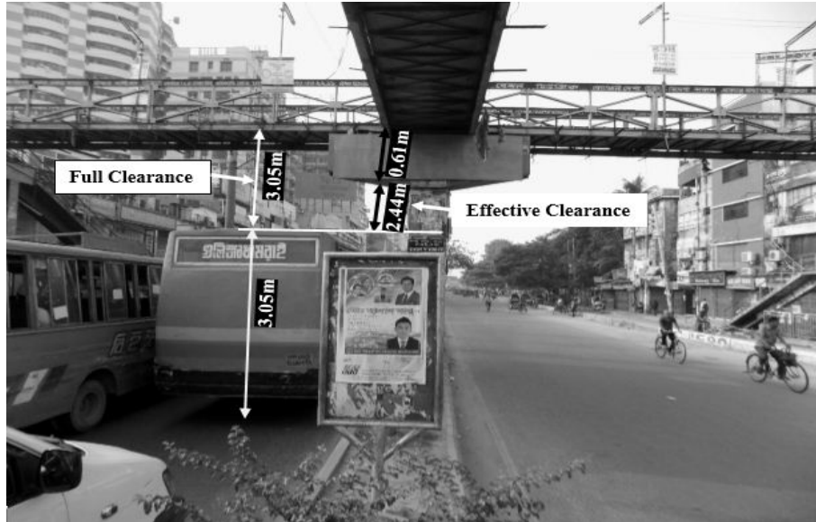
Figure 2: Reduced headroom due to hammer head pier (Science lab Footbridge, Field Survey, 2015)
