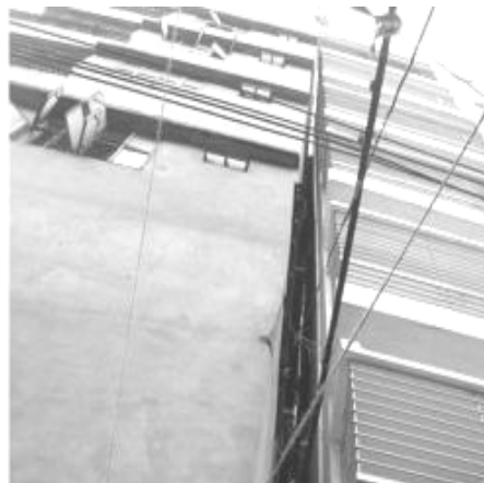
Figure 4: Tilted Building in Bongsal (“Losses of Earthquake”, 2015)
