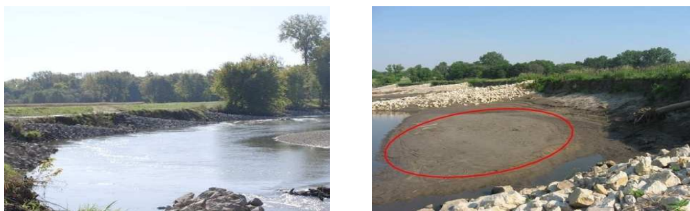
Figure 1: Photographic view shows the series of stream barbs installed along the river bank during flow season (left side) and low flow season (right side). The red circle indicates sand bars formed after installation of barbs.
