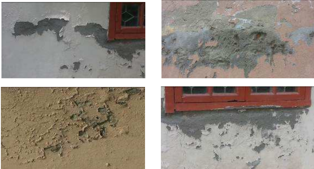
Figure 4: Some picture taken during field survey showing decay of mortar
