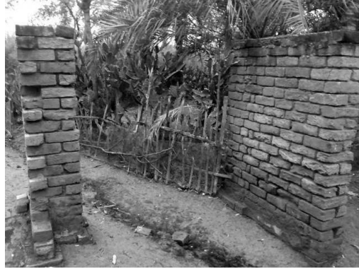
Figure 6: Current status of brick structure due to saline weather
