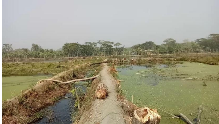
Figure 3: Existing tree is cutdown and root of the trees are removed from the land development site.
