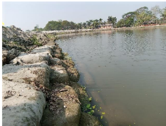
Figure 7: Side protection of lake by use of geo bag in land development site.
