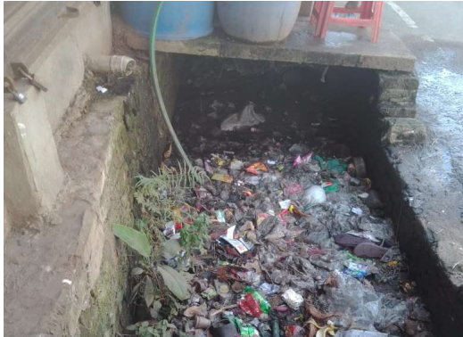
(a) Blockage of the drain due to waste dumping.
