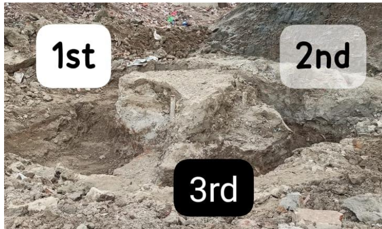
Figure 5: Three Jet Grouted Columns (11m long, approximately 1m diameter and 100mm overlapped)
