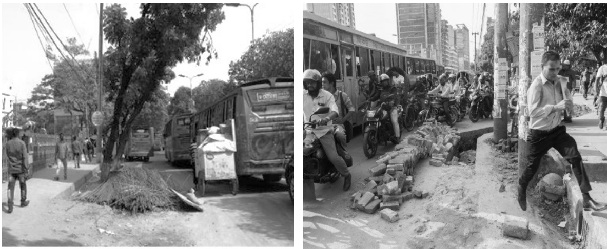
Figure 5: Typical scenarios of exposure of construction and repair materials without adequate protection
