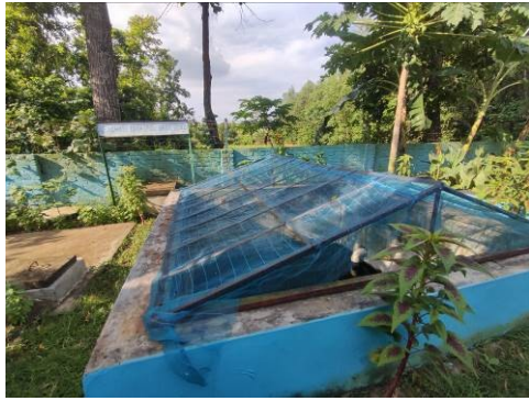
Leachate Tank/ Polishing Pond
