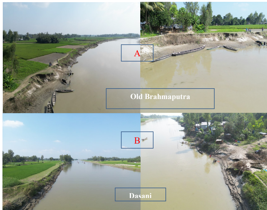
Figure 10: Pictures of Old Brahmaputra (A) and Dasani (B) River bank erosion near at baksiganj upazila in jamalpur district (20/10/2023).
