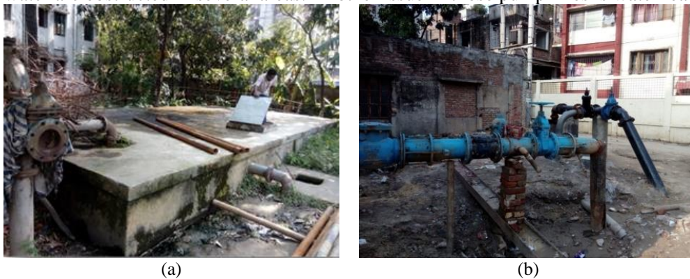
Figure 2: (a) Water reservoir. (b) WASA water pump.
