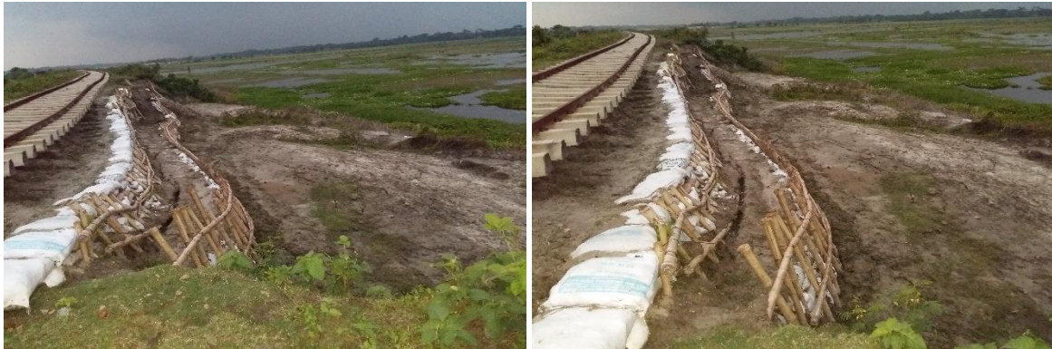
Figure 1: Distressed segment of Railway Embankment
