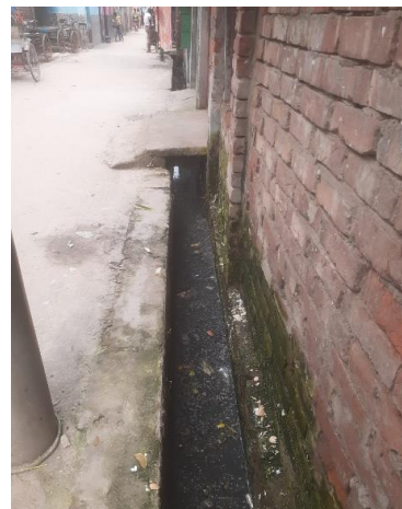
Figure 1 (b): Previous brick drain with ineffective slope and inadequate cross sectional area.
