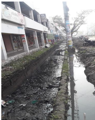
Figure 1(a): Previous drainage system became stagnant due to solid waste disposal.
