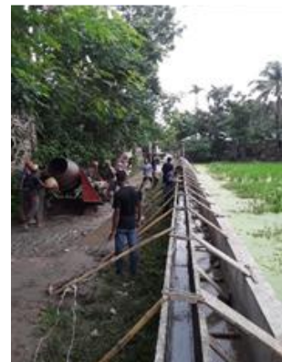
Figure 3 (c): Finishing surface of RCC drain vertical wall after casting at site.
