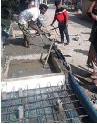
Figure 4 (a): RCC casting of drain top slab is on progress at site.
