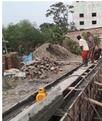
Figure 3 (b): RCC casting of drain vertical wall is on progress at site.
