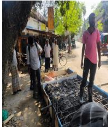
Figure 4 (b): RCC casting of drain top monolithic slab of road crossing structure is on progress
