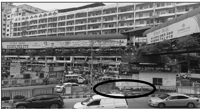
Figure 17. Guard Rails are missing right below Mirpur -1 over bridge.
