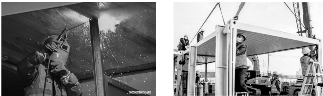
Figure 9: Welding of steel structure (left) (“China Builds New Hospital in 10 Days,” n.d.) On-site, container components are being fastened together in Huoshehsan hospital (right) (Zhou et al., 2020)
