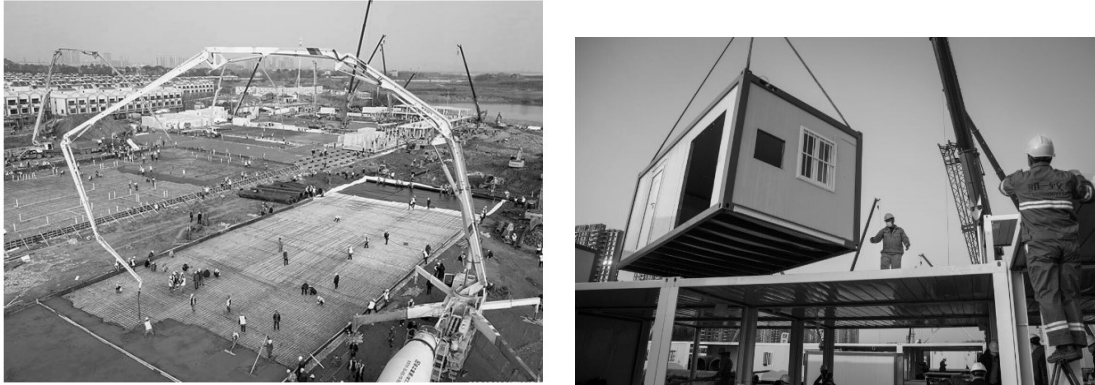
Figure 8: Two days following work, reinforced concrete ground floor slabs were cast in Hoshenshan Hospital (Zhou et al., 2020) (Left); Field Assembly of a Modular Home with a Steel Structure Box Type (“China Builds New Hospital in 10 Days ” n.d.) (Right)
